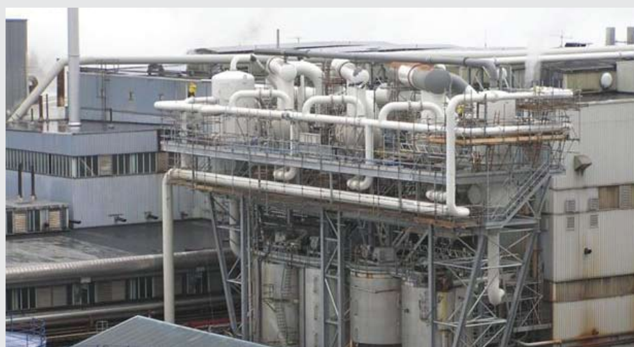
The new pan vapour heaters on the roof of the factory.
