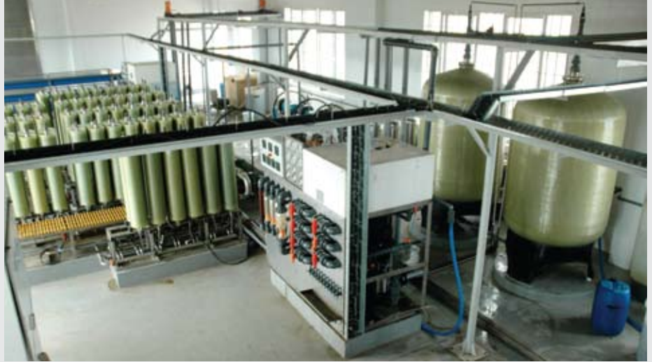
The reverse osmosis ultrafiltration units.
